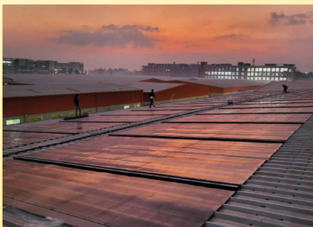
Midsummer is installing a 500 square metre solar roof on a textile factory in Bangladesh.
